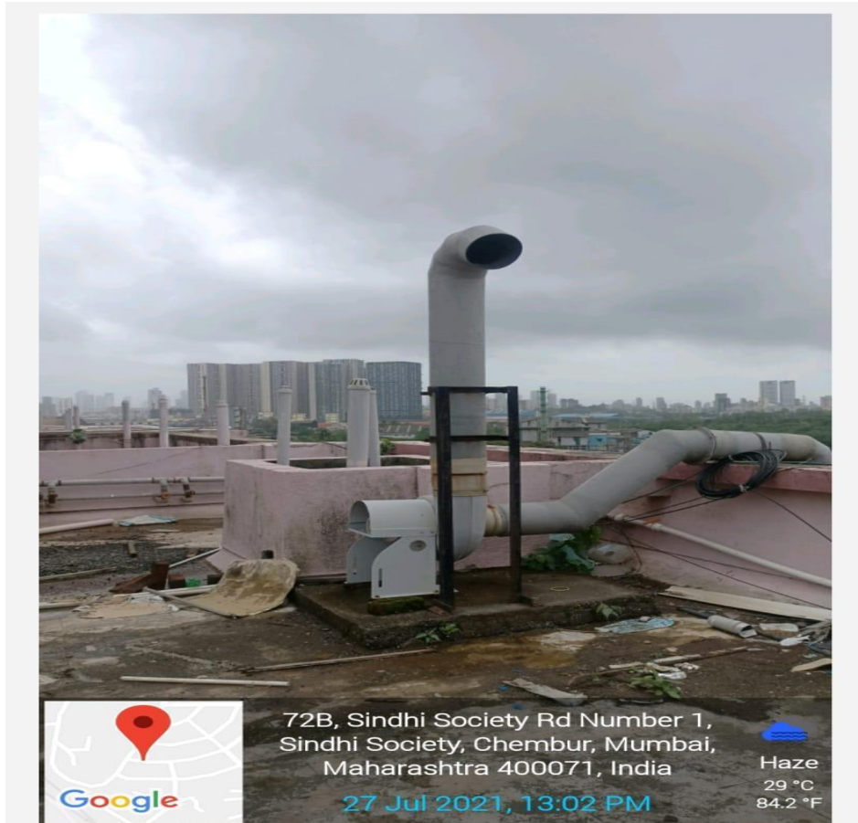
Fig.7.1.3.6. Exhaust of Fume hood installed in VESIT Chemistry Lab
